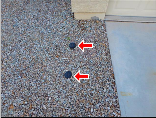
Main Plumbing Clean Outs
