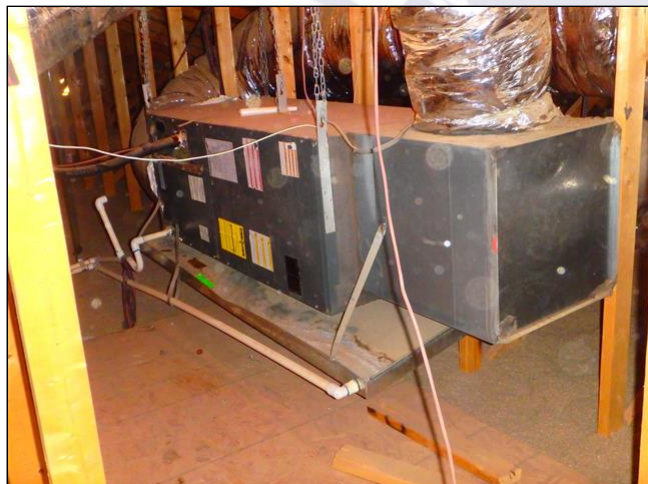
Attic Mounted Air Handler
