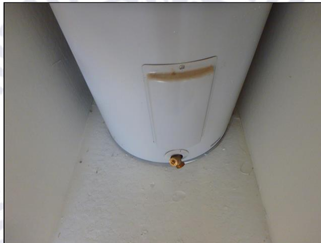
Water heater no leaks
